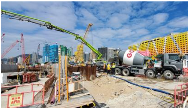
Total of 33 m 3 of material was used to backfill the space between ELS and retaining wall.
