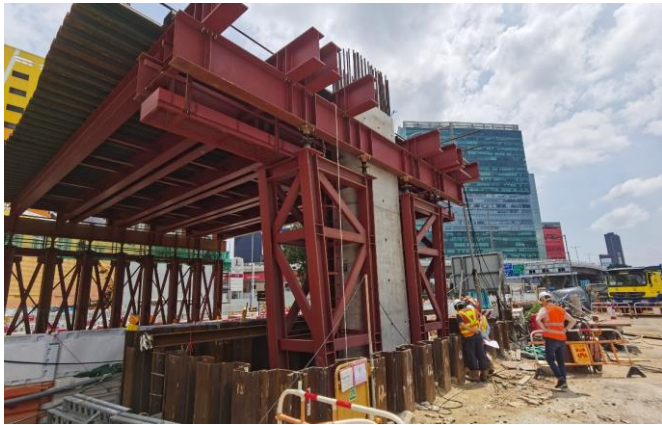
Total of 18 m 3 of material was used to backfill the space between ELS and footbridge pile.
