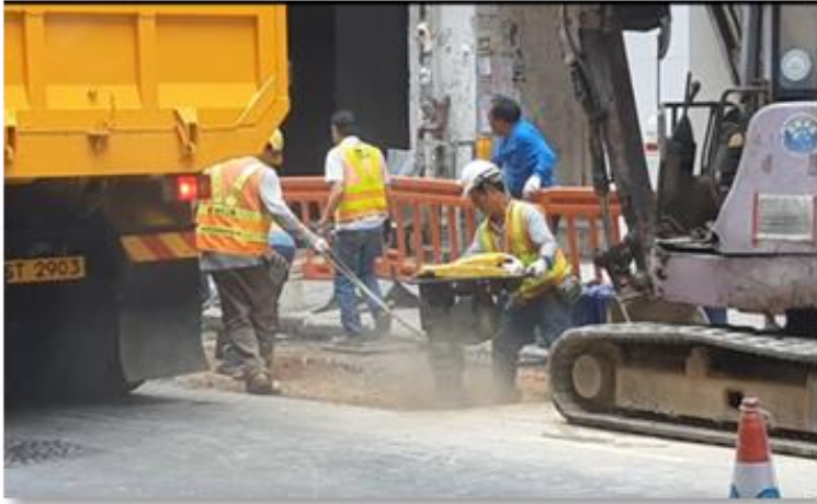
Traditional method of backfilling of soil by mechanical compaction in layer-by-layer method
